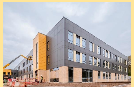
The exterior of our new school building, with the splash of West Coventry Academy gold!
